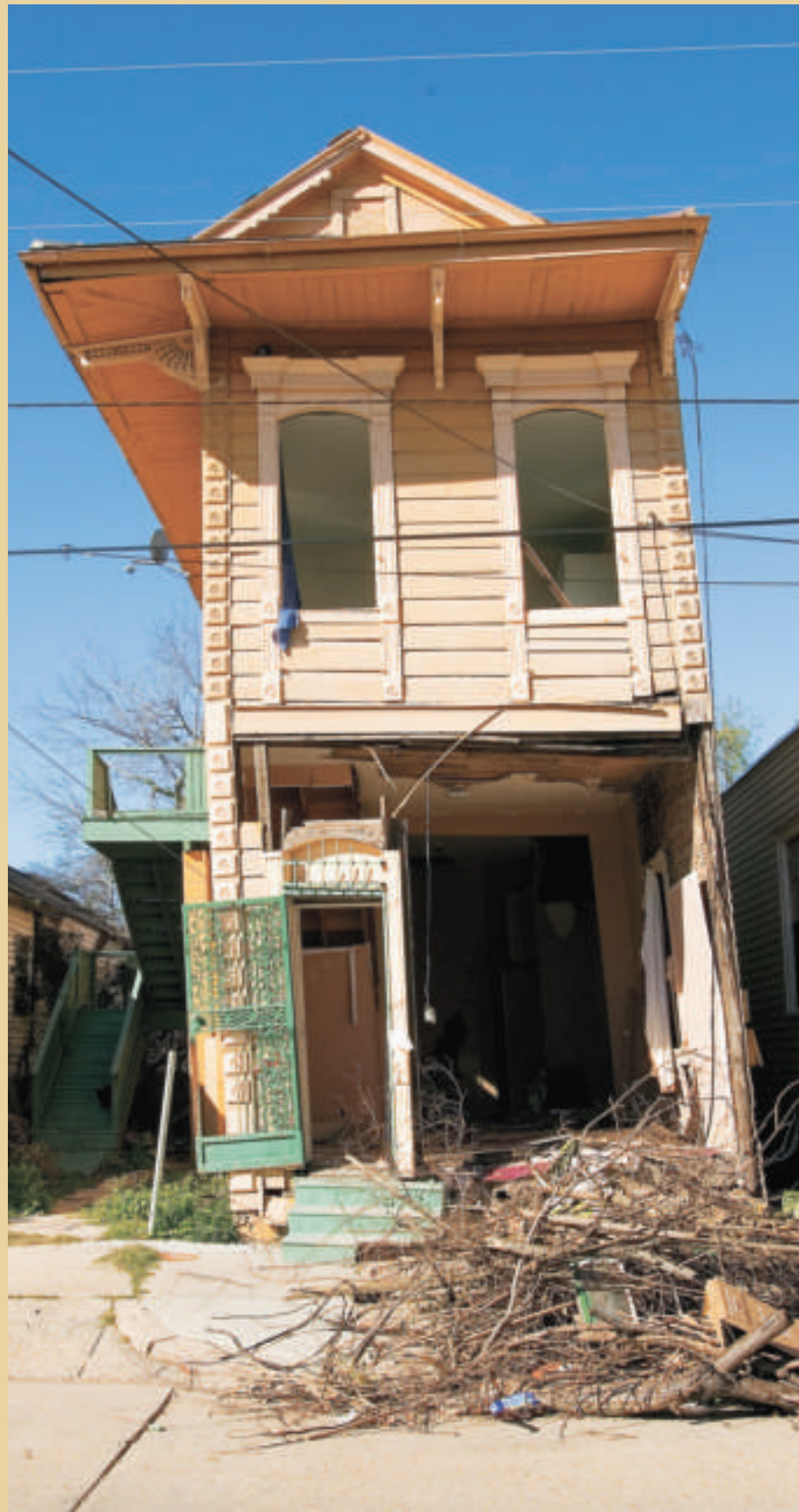
A Victorian-style shotgun house in the Bywater section of New Orleans tilts—the result of Hurricane Katrina's wrath—as if a single push could send it crashing to the ground. The ruined interior and the pile of debris on the sidewalk are common sights throughout the Gulf Coast in the storm's aftermath.
